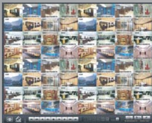
central monitoring system (CMS)
